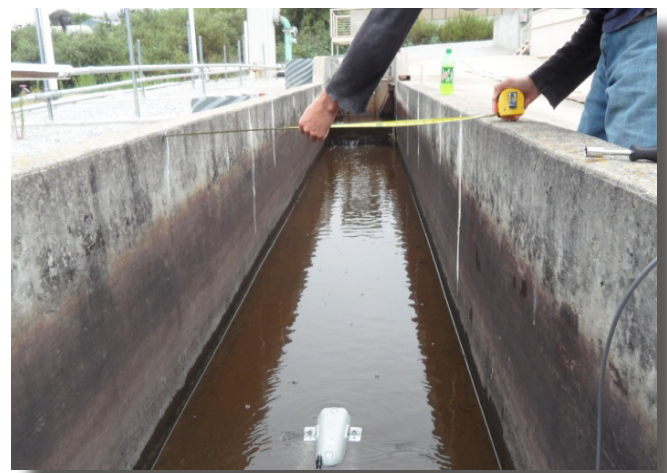
Example of the SonTek-IQ installation in a small canal.
